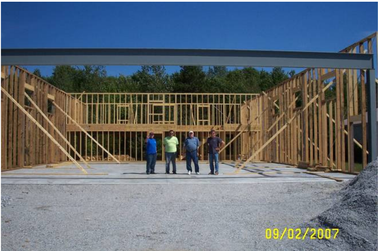
The Hardworking Hangar Bunch (and Tony)
